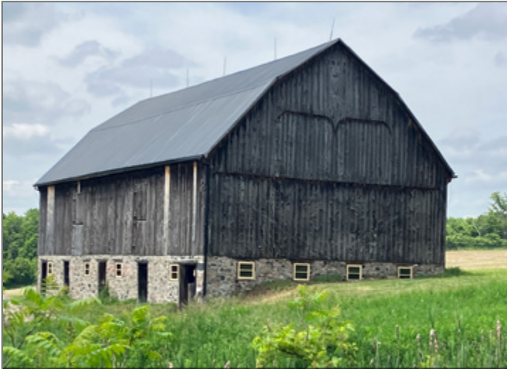
A gambrel-roofed bank barn in admirable condition near Garden Hill. The date “1903” is fretted into the gable boards
